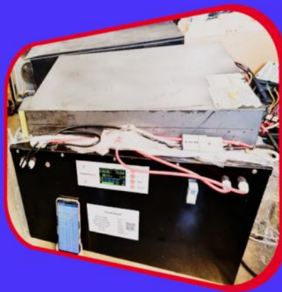
APC 6kva Online UPS 192v 80Ah
